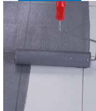
Application of Eco Prim Grip Plus by roller on existing porcelain tiles
